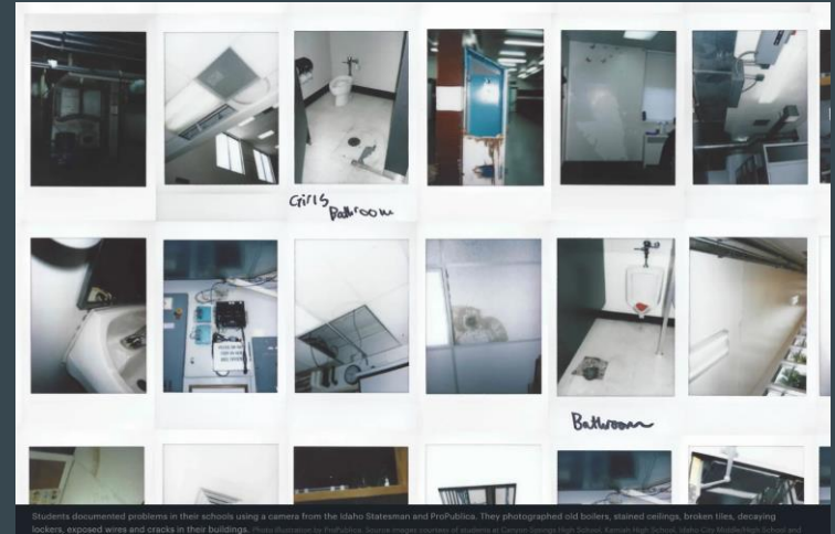
Students documented problems in their schools using a camera from the Idaho Statesman and ProPublica. They photographed old boilers, stained ceilings, broken tiles, decaying lockers, exposed wires and cracks in their buildings. Photo courtesy of ProPublica. Source: Images courtesy of students at Canyon County High School, Canyon High School, Idaho City Middle High School and
