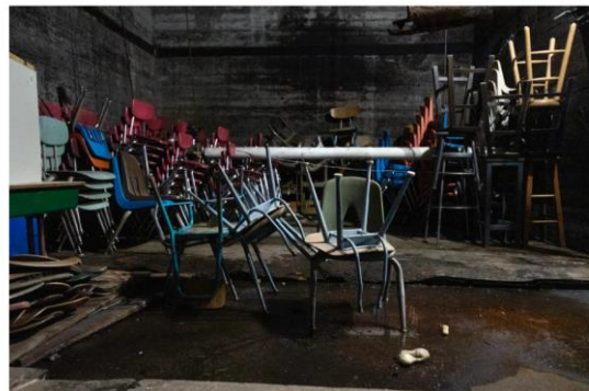
Water seeps across the floor in the boiler room at Valley View Elementary School in Bonners Ferry, Idaho. The aging school is part of the Boundary County School
